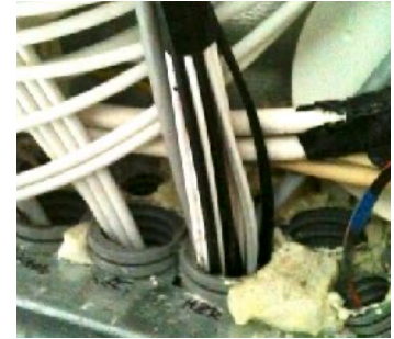
In 2011, nine POF cable-strands were pulled from the basement to the first floor using only two empty tubes of the ductwork.
