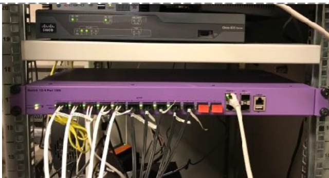
The existing POF-cables were simply connected to the new Homefibre gigabit smart switch, just with fresh cut cable heads.
